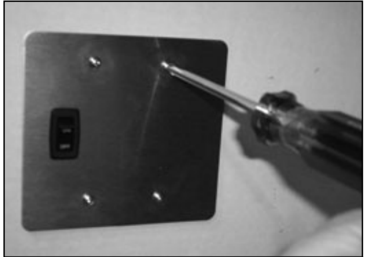
Figure 12.9 Switch Cover Plate
